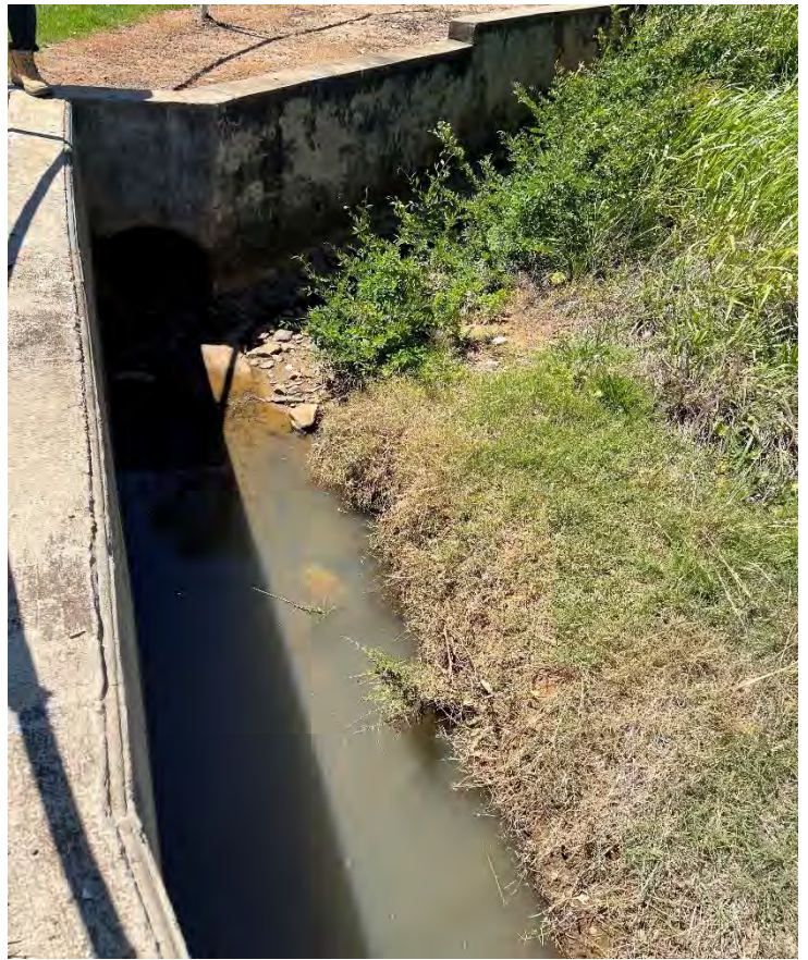
Figure 16 Water ponding in drainage channels
