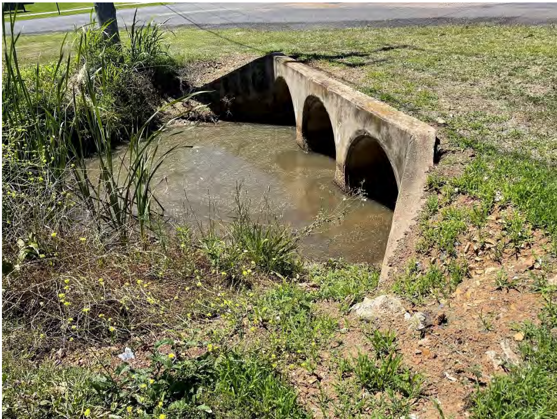
Figure 11 Water ponding downstream of channel
