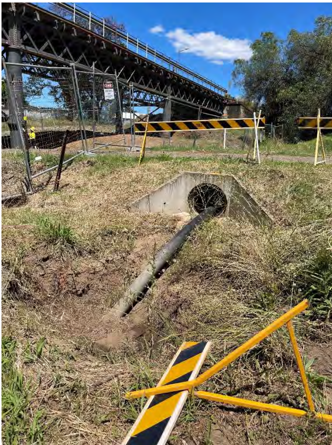
Figure 17 Outlets to Namoi rivers with water pipe within pumping water out of river
